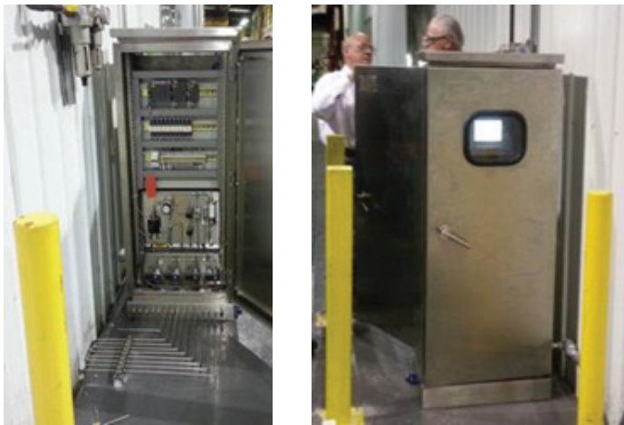
Figure 5. CDU block of a multi-point system, installed in general-purpose area indoors, but outside the monitoring area.
