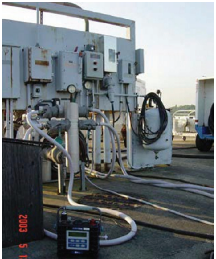
Figure 4. AreaRAE monitoring mechanical equipment.
