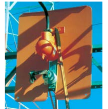
Barrier and switch jaw guard installed on a substation switch.
